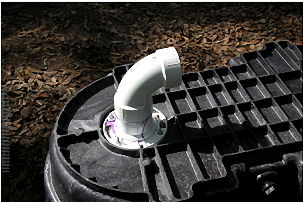
Photo 6: Installed sludge drain
